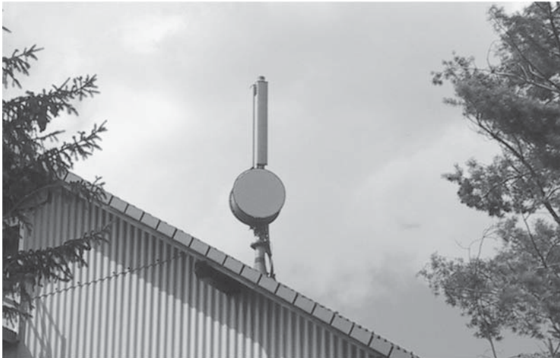
Figure 1.19 A typical antenna of a GSM base station. The optional microwave directional antenna (round antenna at the bottom of the mast) connects the base station with the GSM network. Reproduced by permission of Martin Sauter.
